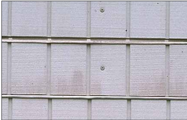
Figure 16–16. Demonstration of proper and improper z-flashing installation: (top) siding installed with a 9-mm (3/8-in.) gap between the z-flashing and siding to allow water to drain off the siding; (bottom) siding installed without a gap, which gives easy access for water absorption into the siding and thus shows extractives staining.
