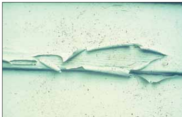
Figure 16-23. Intercoat peeling of paint, usually caused by poor preparation of old paint surface or excessive weathering of primer prior to application of top coat.
